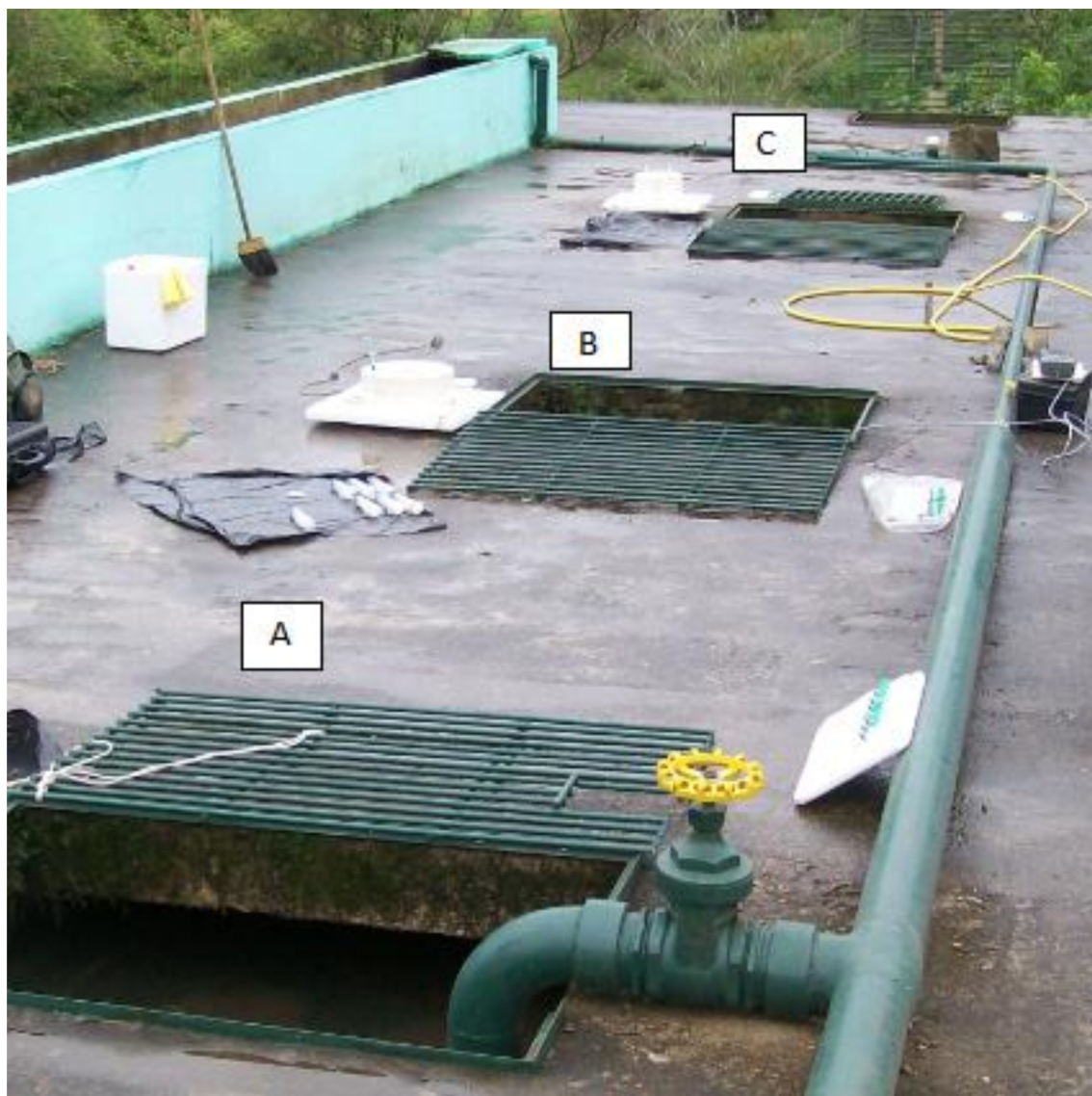
Figure 1S. The covered aeration tank of the wastewater treatment plant and the openings (A, B and C) through which all measurements were made
